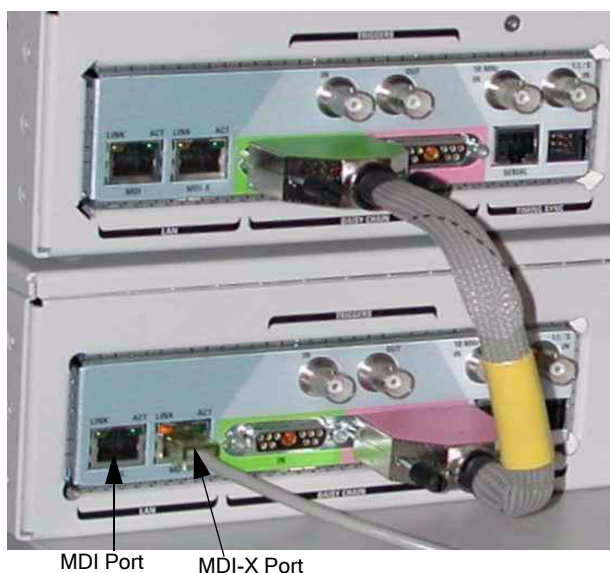
Figure 9 Interconnection between the Master and Slave Chassis
